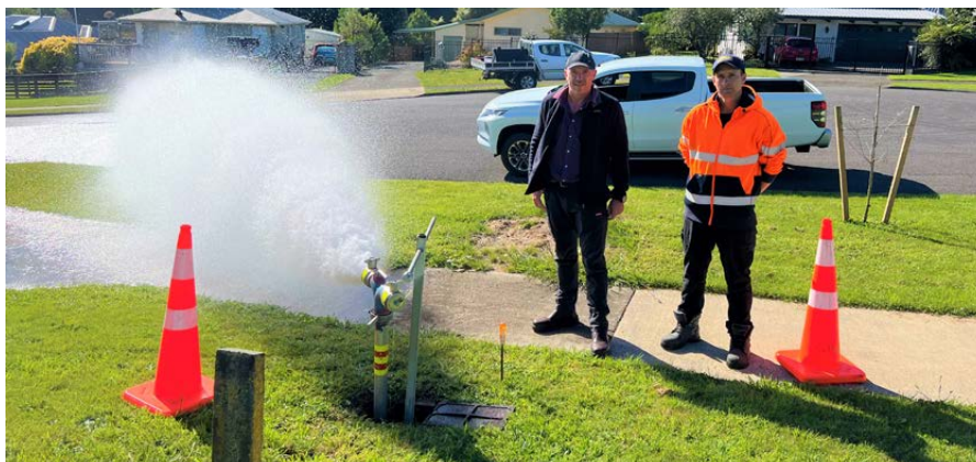
Engineering Manager, Operations and Services Riaan Nel (left) and Team Leader, Three Waters Glen Penny examining the increased water pressure flow from a hydrant stand as it flushes the lines.
