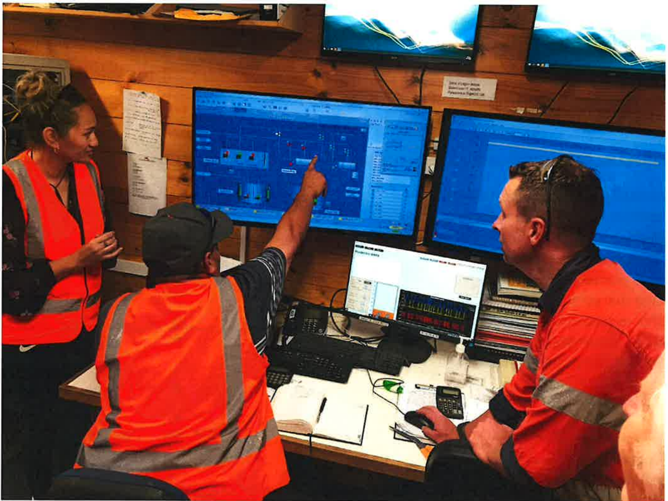
Mayor Faylene Tunui and Deputy Mayor view the new telemetry operations system installed at the Waste Water Treatment Plant control room with Three Waters Team Leader Glen Penny.
