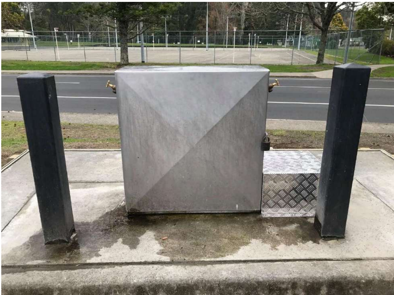
WATER STATION AT NEW WORLD CARPARK
